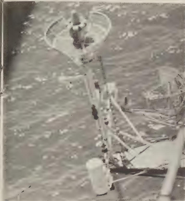
The intercept and direction-finding antenna of an Italian INS-3 installed on the Indian frigate Godavari , 1986.
